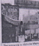
The entrance to Gandhi Memorial Hall is being widened to improve its visibility from the road.
